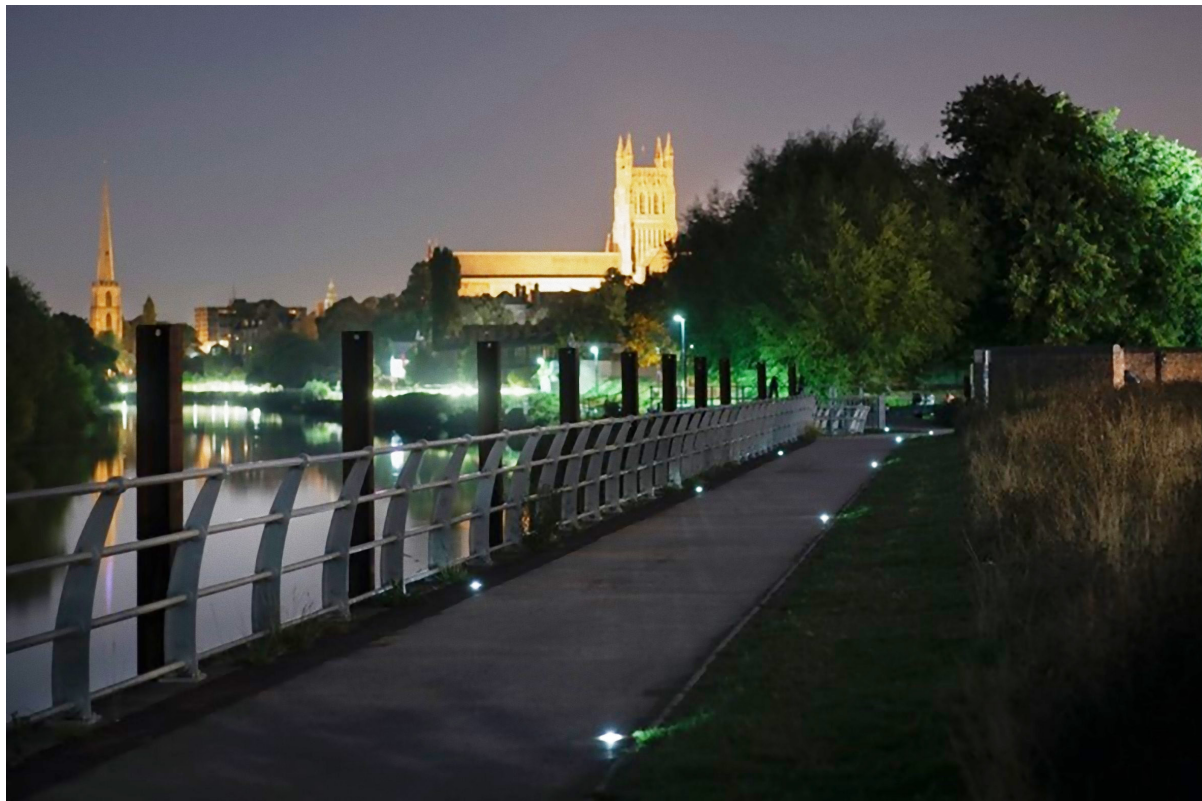
Photo 5: Ground-mounted, solar-powered, cowled, way-markers installed in the green infrastructure of a residential development near Worcester Cathedral.
